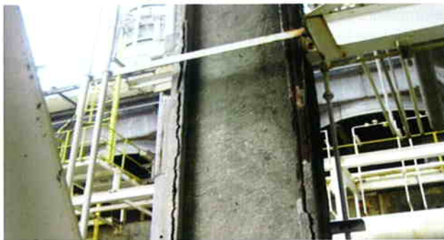
Figure 4: Structural cracks in concrete fireproofing
