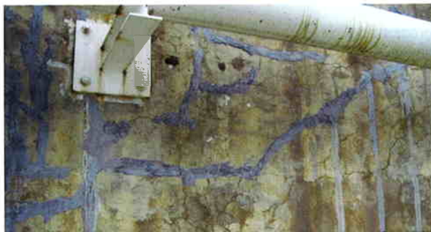
Figure 5: Structural cracks due to vibration
