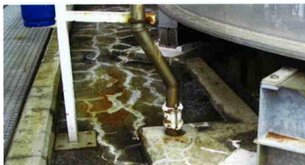
Figure 6: Widespread structural cracks
